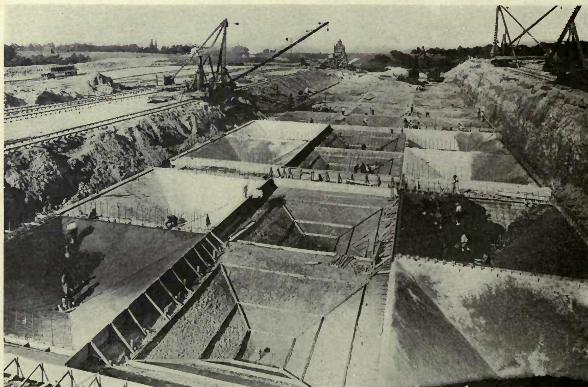
Rochester Sewage Disposal Plant, Rochester, N. Y.
